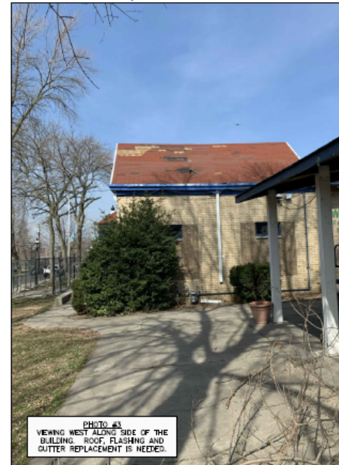
PHOTO #4 VIEWING NORTHWEST ALONG THE BUILDING FRONTAGE WINDOW REPLACEMENT IS NEEDED.
