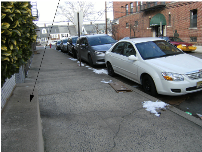
VIEW OF SIDEWALK IN FRONT OF WEST 17TH STREET LOOKING TOWARDS JFK BOULEVARD
